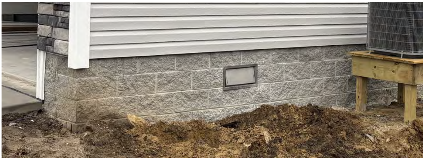
ENGINEERED FLOOD VENT IN SIDE OF GARAGE
