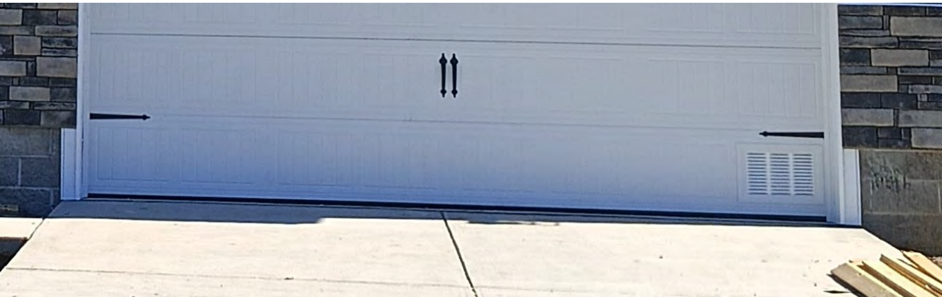
NON-ENGINEERED FLOOD VENT IN GARAGE DOOR
