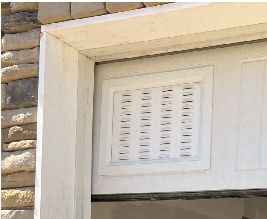
NON-ENGINEERED FLOOD VENT IN GARAGE DOOR
