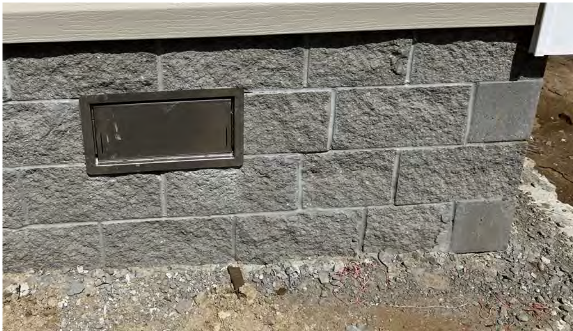
FLOOD VENT IN SIDE OF GARAGE
