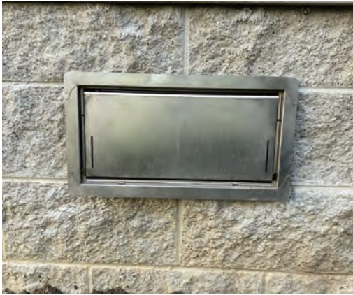
ENGINEERED FLOOD VENT IN SIDE OF GARAGE FOUNDATION
