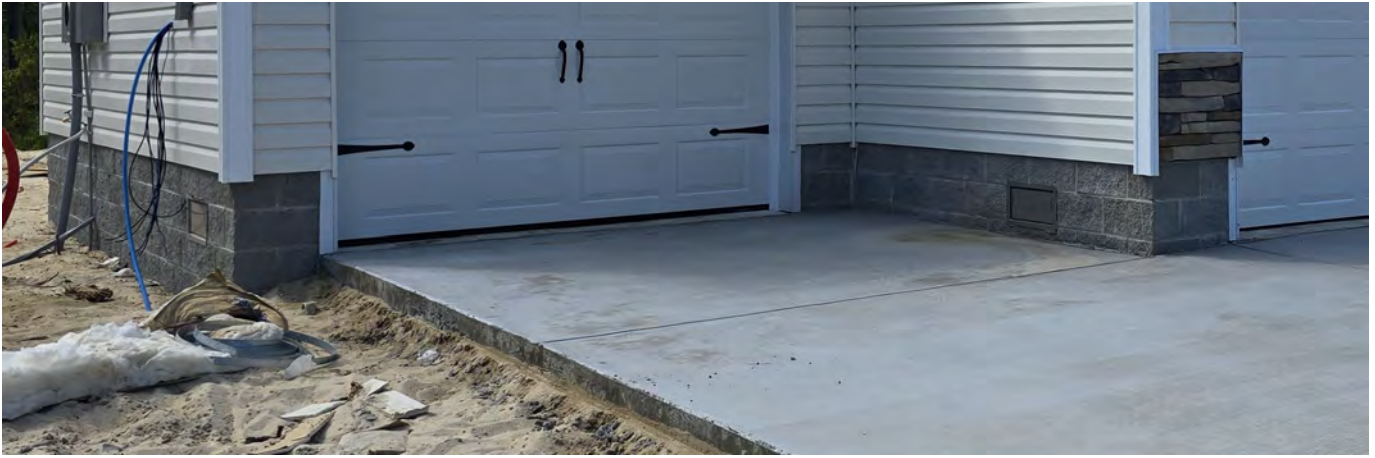
ENGINEERED FLOOD VENTS IN GARAGE
