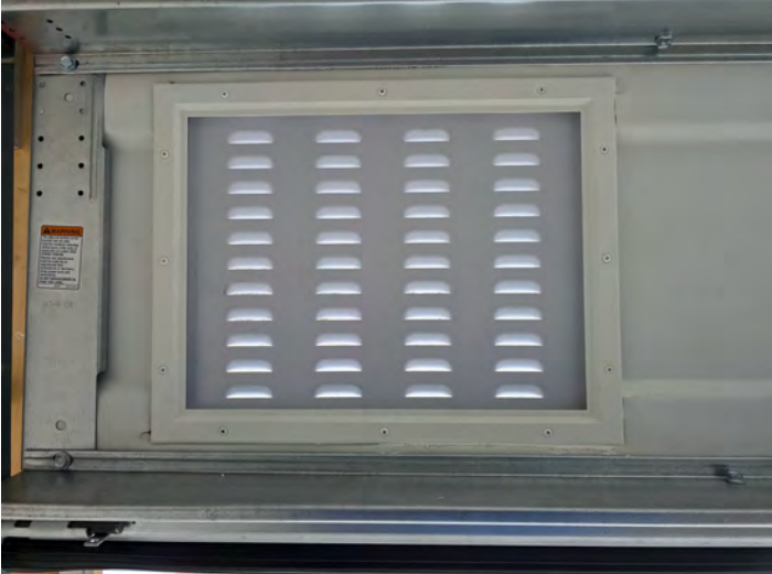
NON-ENGINEERED FLOOD VENT IN GARAGE DOOR - REAR
