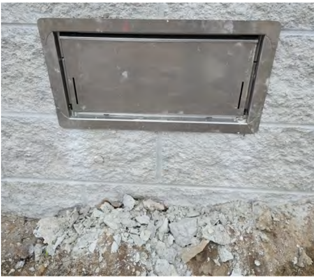
ENGINEERED FLOOD VENT IN SIDE OF GARAGE
