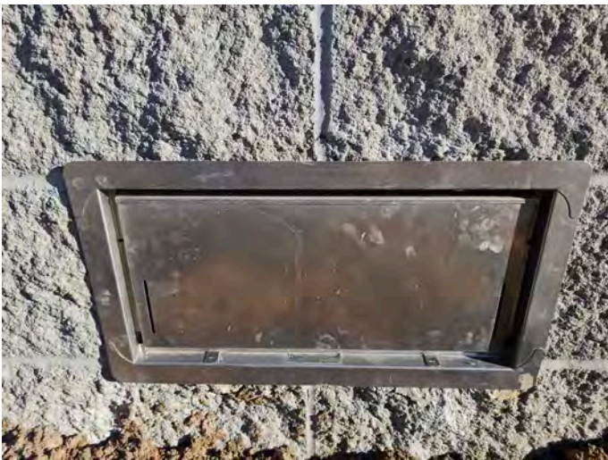
ENGINEERED FLOOD VENT IN SIDE OF GARAGE FOUNDATION
