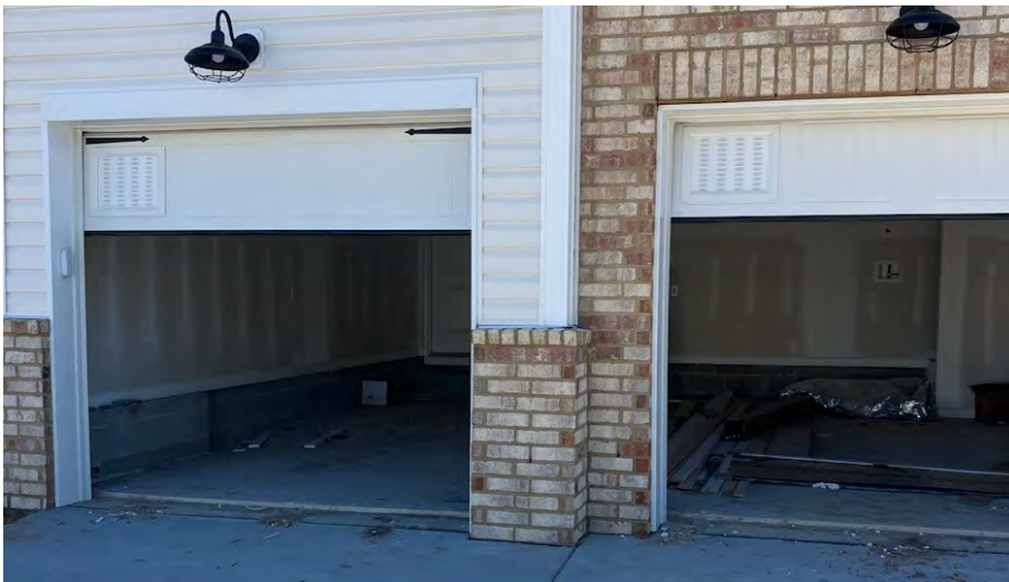
NON-ENGINEERED FLOOD VENTS IN GARAGE DOOR
