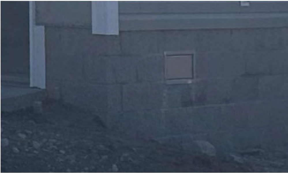
ENGINEERED FLOOD VENT IN SIDE OF GARAGE
