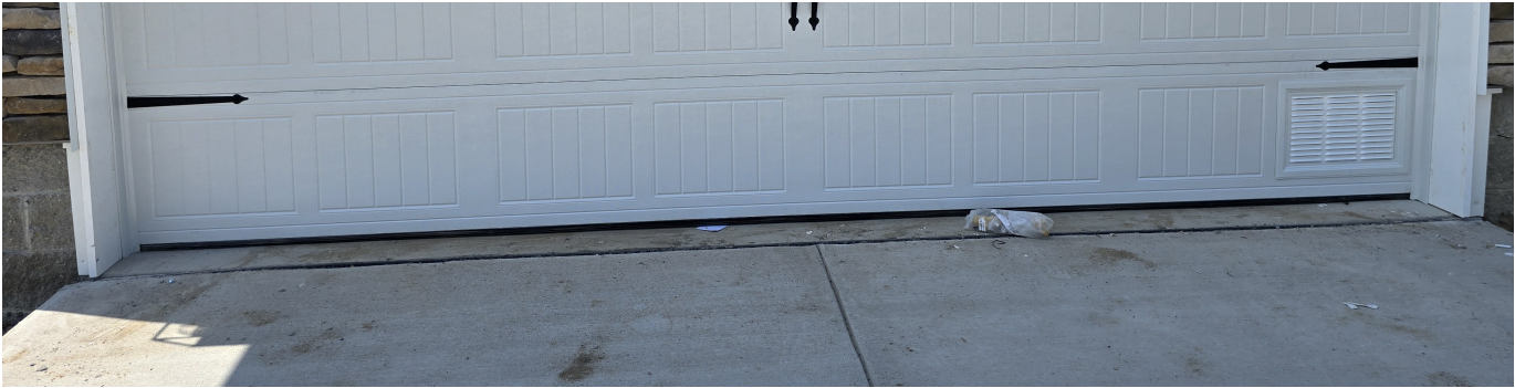
NON-ENGINEERED FLOOD VENT IN GARAGE DOOR
