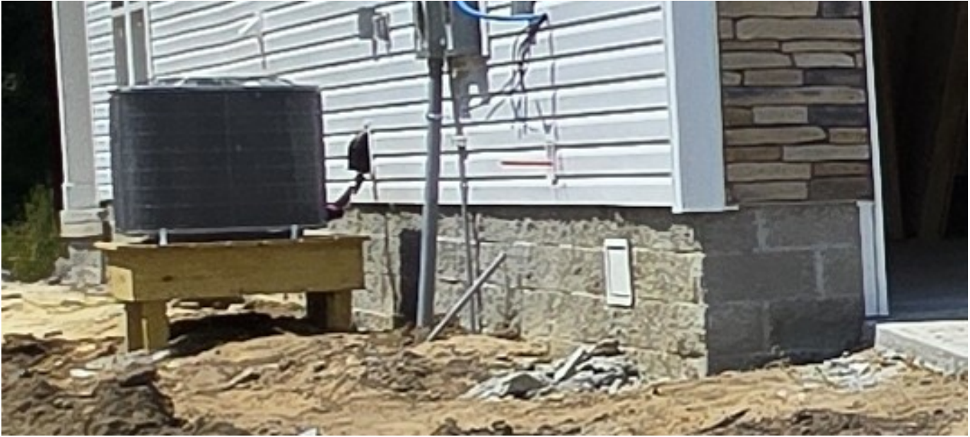
ENGINEERED FLOOD VENT IN SIDE OF GARAGE
