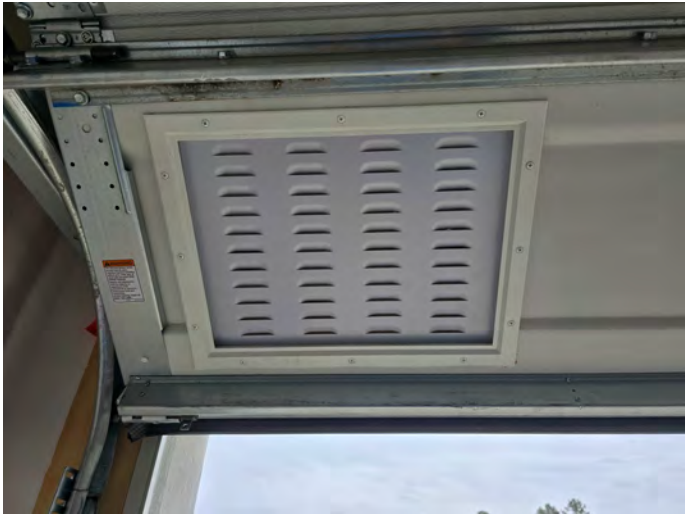
NON-ENGINEERED FLOOD VENT IN GARAGE DOOR (BACK)
