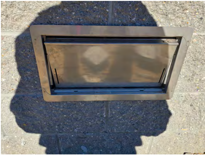
ENGINEERED FLOOD VENT IN SIDE OF GARAGE
