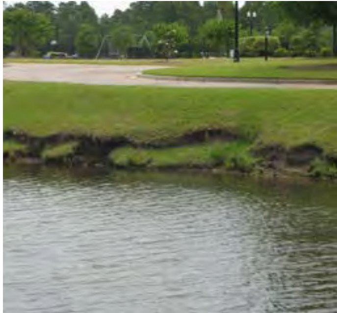
Pond Bank Erosion Source: Clemson Extension, n.d.
