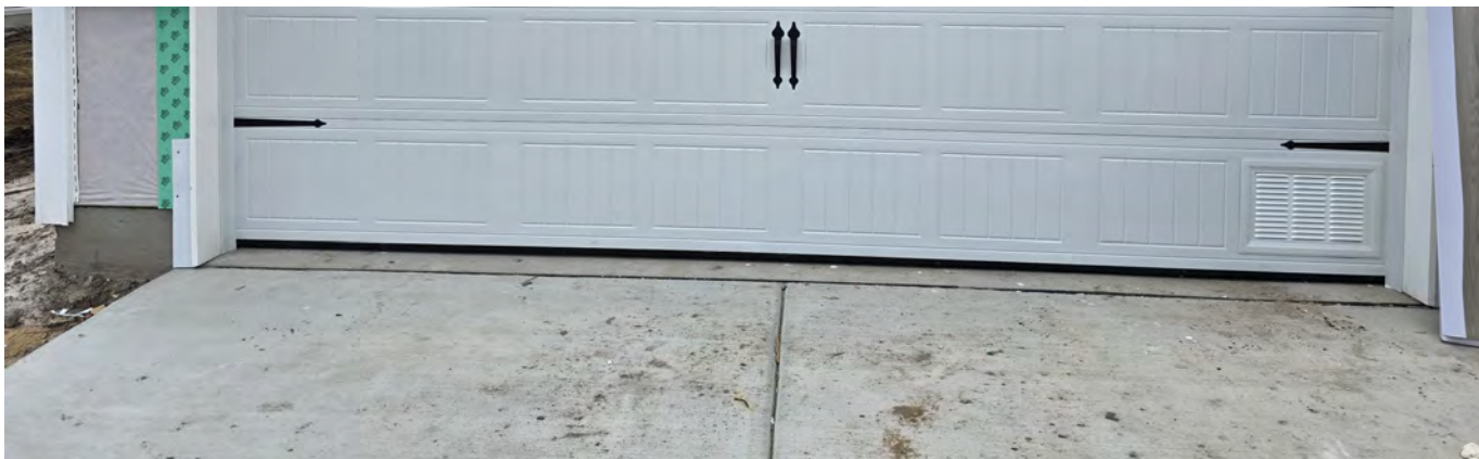
NON-ENGINEERED FLOOD VENT IN GARAGE DOOR
