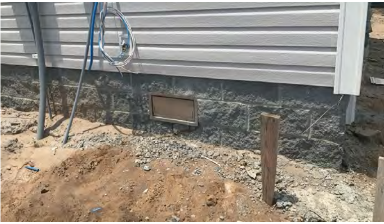
ENGINEERED FLOOD VENT IN SIDE OF GARAGE
