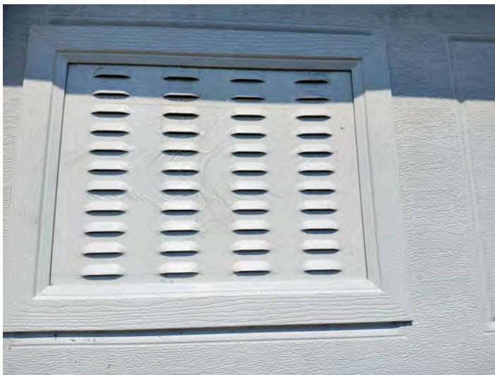
FRONT OF NON-ENGINEERED FLOOD VENT IN GARAGE DOOR
