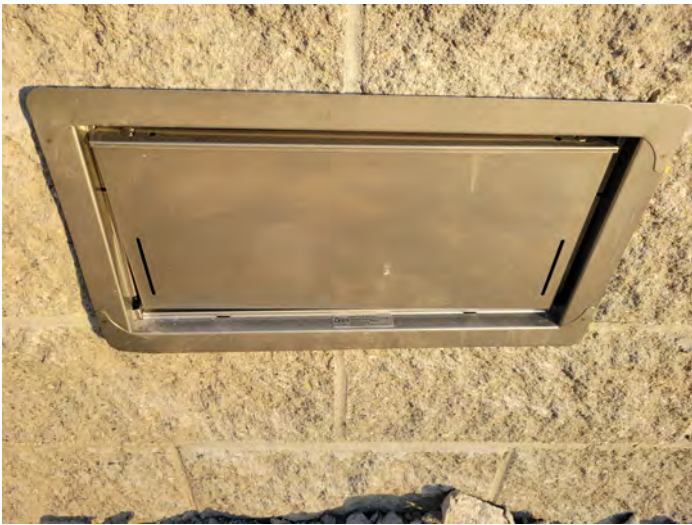
FLOOD VENT IN SIDE OF GARAGE
