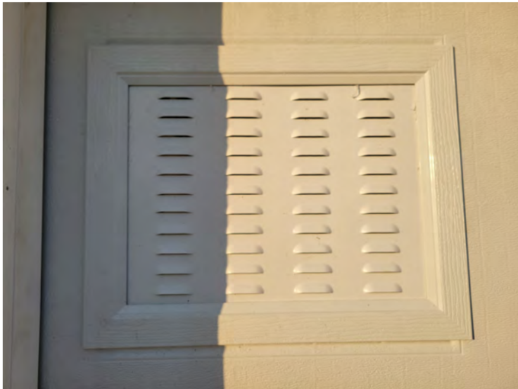
NON-ENGINEERED FLOOD VENT IN GARAGE DOOR
