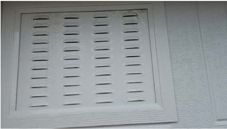
NON-ENGINEERED FLOOD VENT IN GARAGE DOOR
