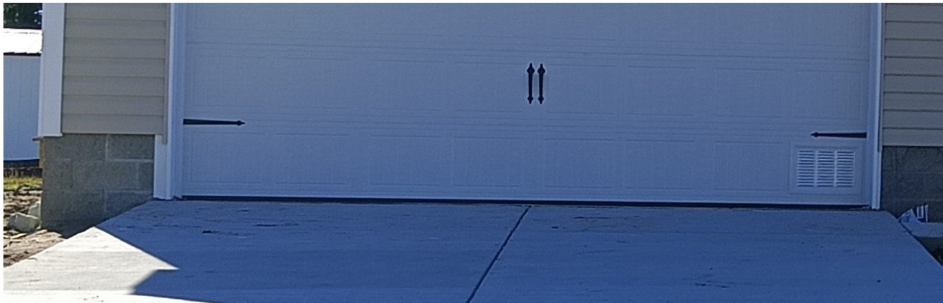
NON-ENGINEERED FLOOD VENT IN GARAGE DOOR
