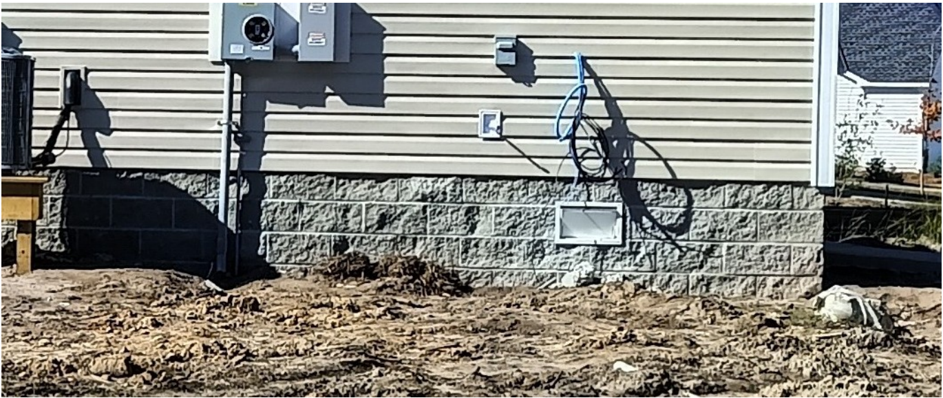
ENGINEERED FLOOD VENT IN SIDE OF GARAGE
