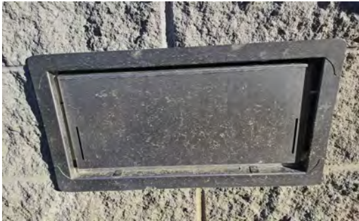
ENGINEERED FLOOD VENT IN SIDE OF GARAGE FOUNDATION
