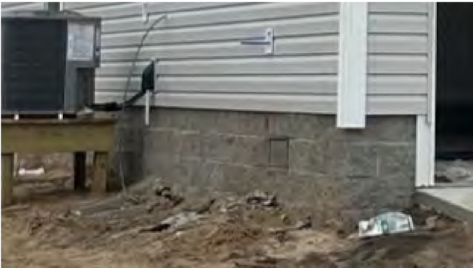
ENGINEERED FLOOD VENT IN SIDE OF GARAGE
