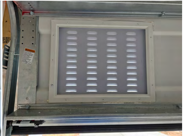
NON-ENGINEERED FLOOD VENT IN GARAGE DOOR (BACK)
