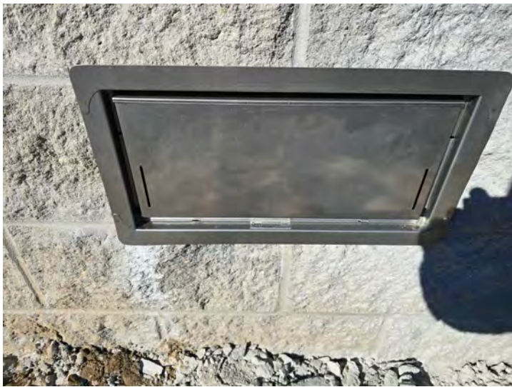
ENGINEERED FLOOD VENT IN SIDE OF GARAGE
