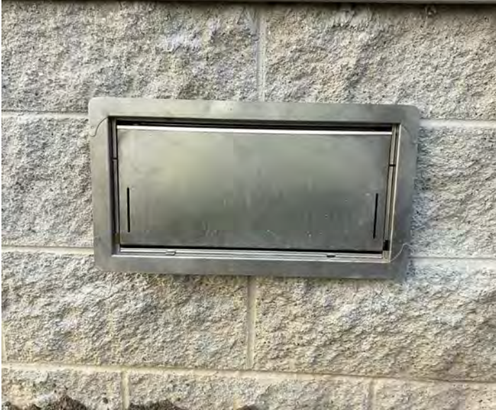
FLOOD VENT IN RIGHT SIDE OF GARAGE
